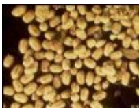
drywood termite fecal pellets
